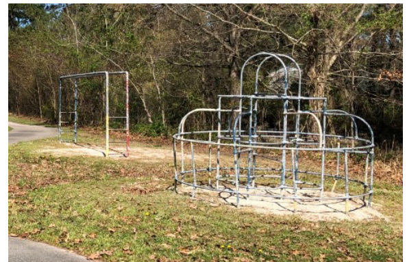
Poplar Hall Park - Aging play equipment on substandard playground safety surfacing and extents
